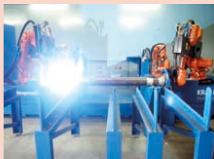
4. The flanges are then fitted and tacked to the pipe using two of the robotic arms
