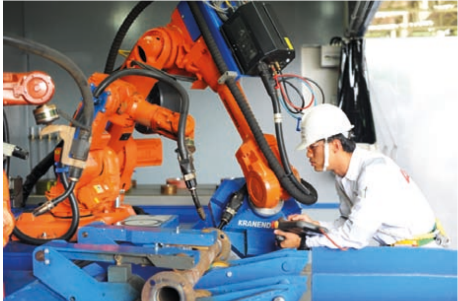
Keppel Singmarine is in the process of incorporating robotic applications to its steel cutting and fabrication processes
