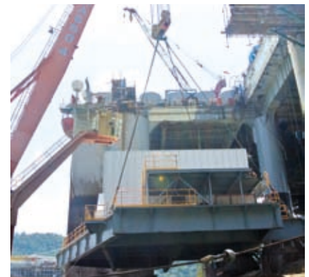
Despite the complex task of lifting the 240 metric tonne living quarters onto the semi Ocean Quest, the BrasFELS team was able to think of an innovative solution and complete the lifting operation in just 10 days
