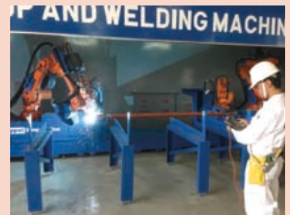
5. Finally, the flanges are welded to the pipe using all four robotic arms simultaneously
