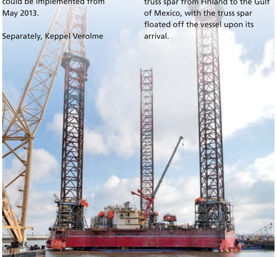
Keppel Verolme utilised to good effect the JUMP system, a new technology jointly developed with Austrian company Palfinger, to access and work on the rig legs of Ezion Holding's jackup Prime Exerter
